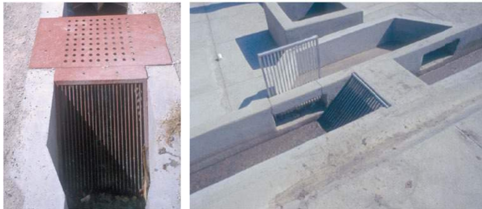
Figure 28.h. Typical Bar Screen Installations
